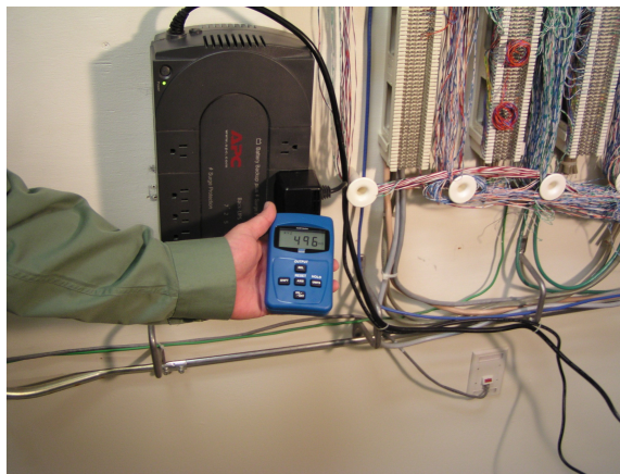
Example of ELF radiation located in a typical telephone switching room and how to detect it
